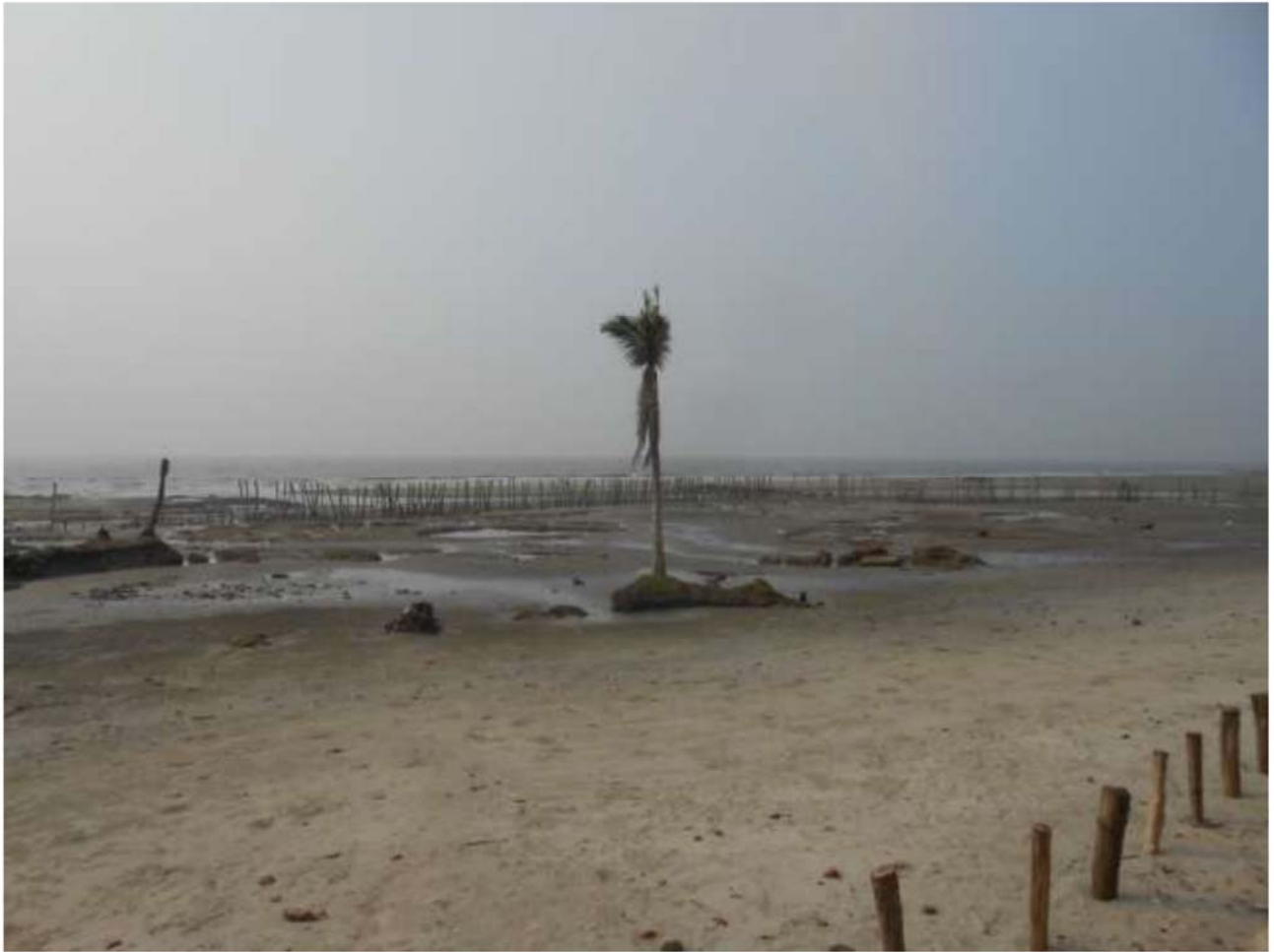
Plate 162 – Shibpur Boatkhal area in the South Eastern Coast. There is a huge coastal erosion in this part of the island 21^{\circ}38'3.28''N 88^{\circ}7'15.94''E
