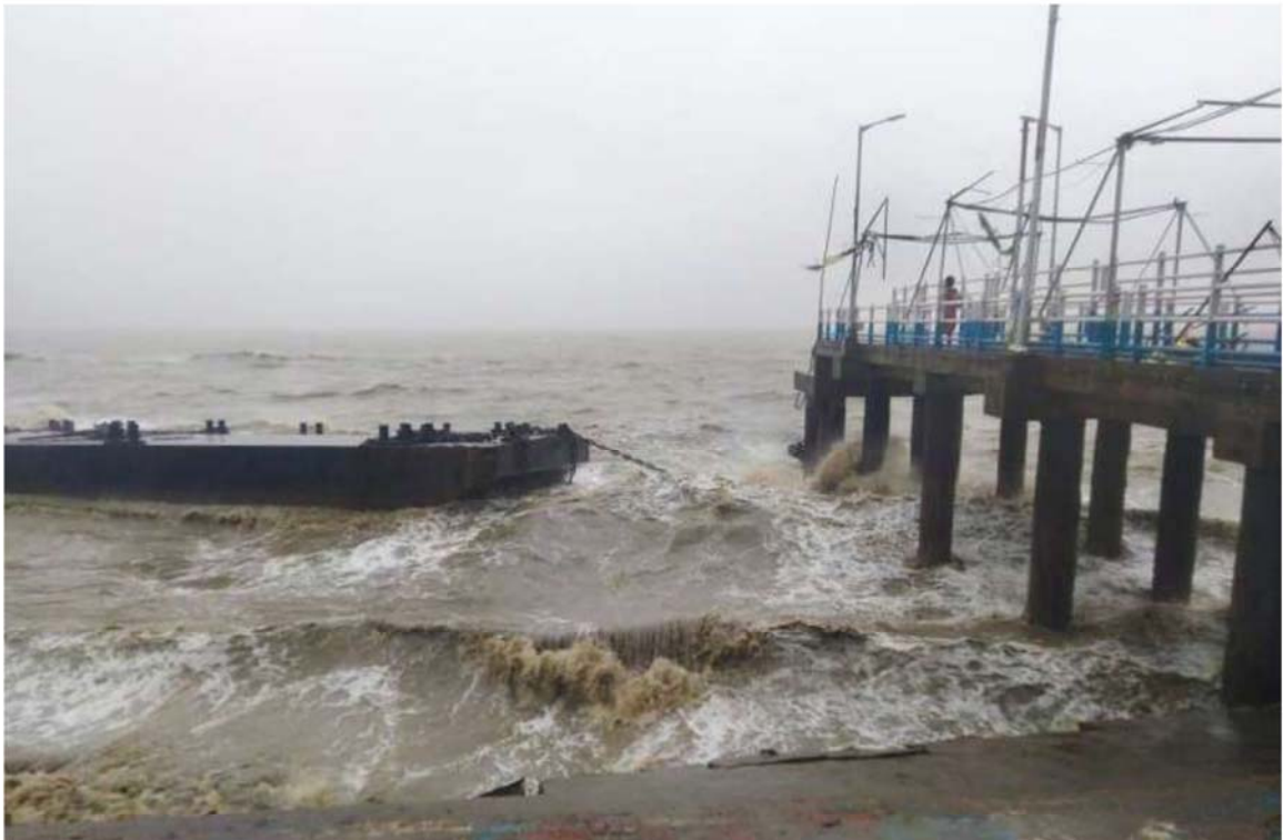
Plate 150– March 26, 2020 . Kochuberia Jetty got dismantled due to Cyclone Amphan, Source -
