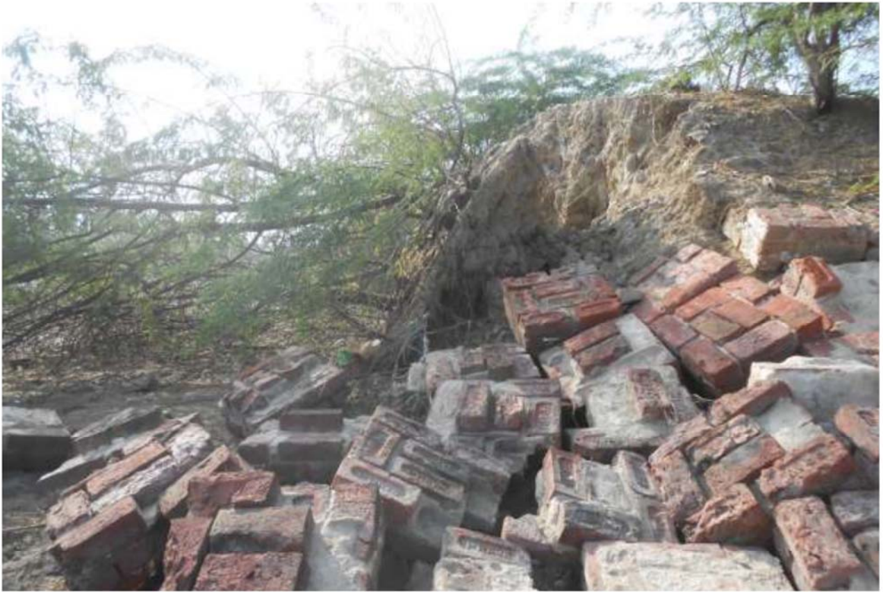
Plate 160– Broken Embankment , Baliary , Moushuni Island
