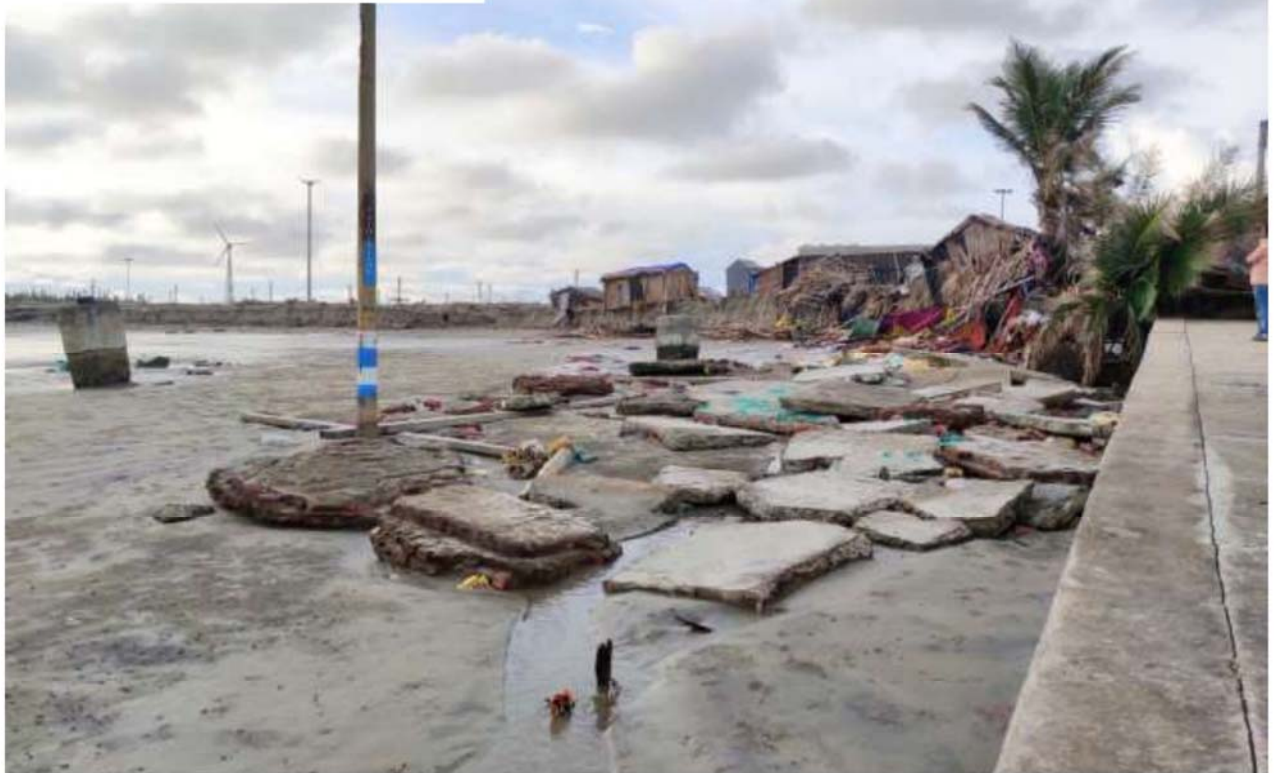
Plate 158 – Ganga sagar Beach , Broken Beach Embankment
